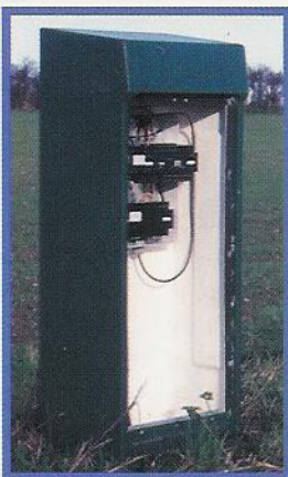
A remote RTU station: it shouldn't depend on mains power
