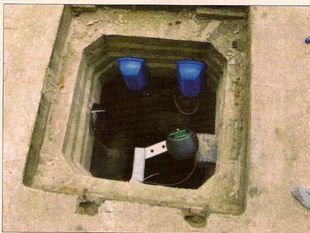
An ATEX compliant wireless device is installed in a potentially explosive atmosphere to monitor the site and report incidents.
